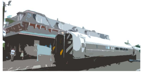
Wallingford's new train station is under construction and commuter rail service is expected to begin by the end of 2016.
